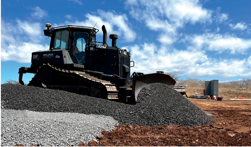
A Cat D6 dozer at Goodfellow's Kihei High School project PHOTO COURTESY: GOODFELLOW BROS.
